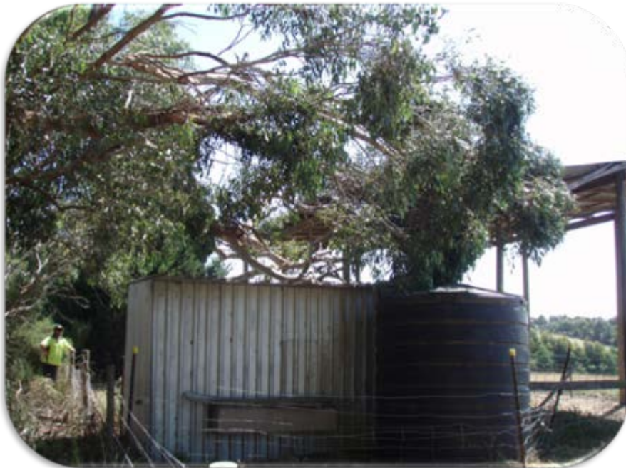
Damage to Private Property from Council Tree
