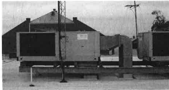
Main air conditioning units for extension section (viewed from 1 st floor roof)
