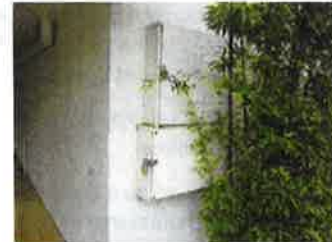
Photo: Outdoor Metering Enclosure
