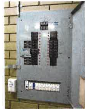
Photos: Curves Switchboard
