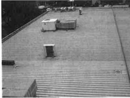
Main air conditioning units for original section (viewed from 1 st floor roof)
