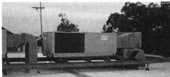
Main air conditioning units for new section (viewed from 1 st floor roof)
