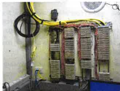
Photo: Main Distribution Frame
