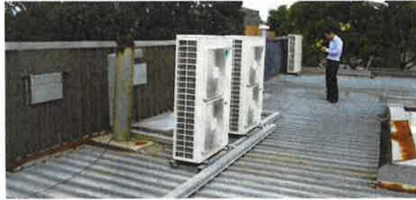
Carino's Building – Three air conditioning units for main office area (photo above) and two more air conditioning units for main office area (photo below) (all condensing units on roof) N.B. some capping on the top of the walls is quite rusted.
