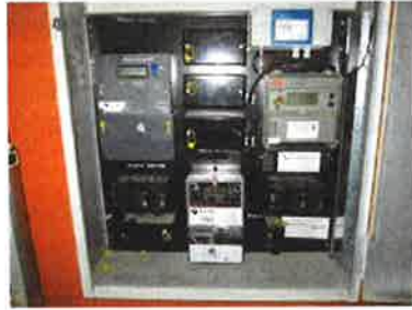
Photo: Main Switchboard with Metering
