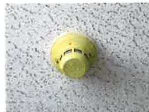
Photo: Smoke Detector (Unknown manufacture)
