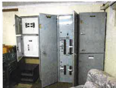
Photo: Main Switchboard
