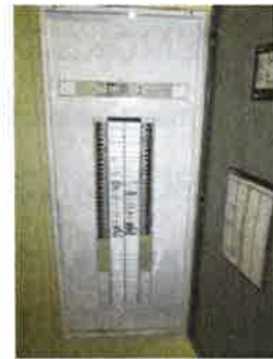
Photo: Carino's Main Switchboard
