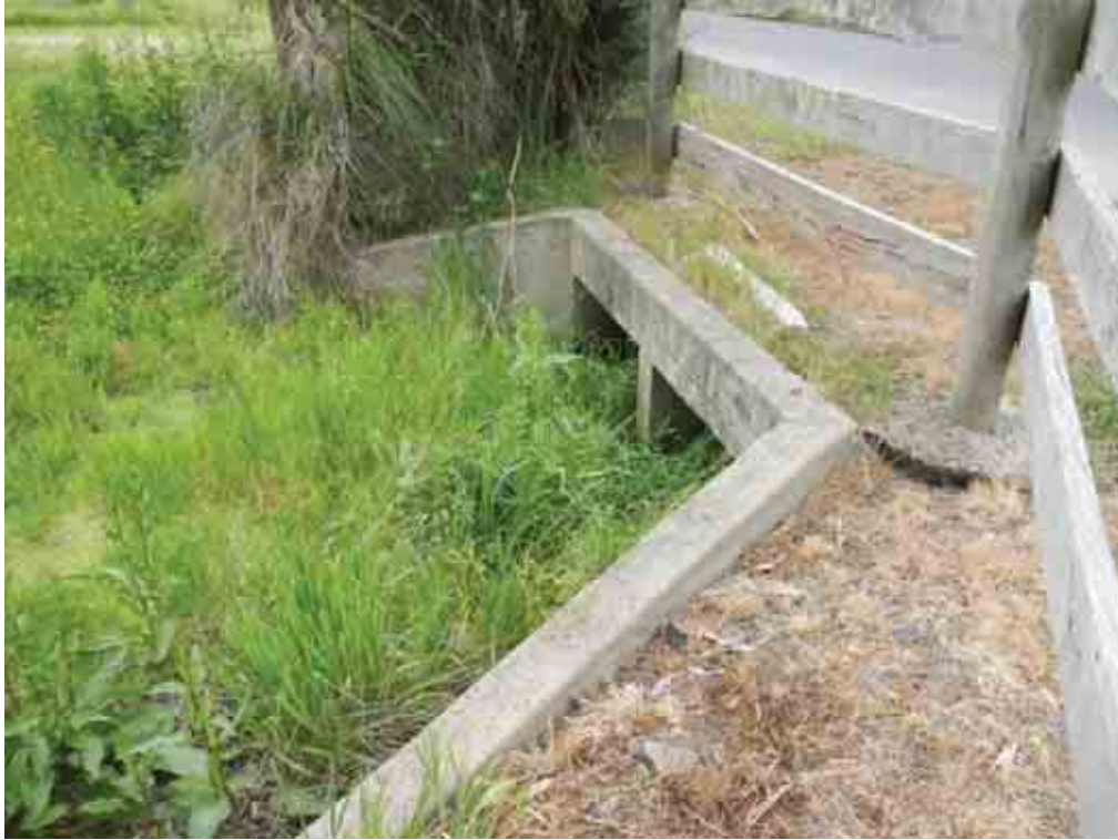
Figure 3.5 View north to the inlet of the 2 no. 1200 mm wide by 600 mm high box culverts located under Follett Drive
