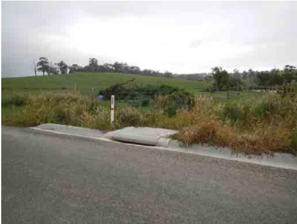
Figure 3.7 View west to new side entry pit and kerb and channel on Henrys Road near the intersection with Eagle Rise.
