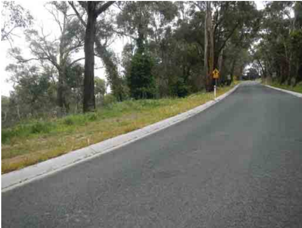
Figure 3.8 View north on Henrys Road showing new kerb and channel and road reconstruction works
