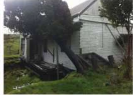
Damage to house due landslip
