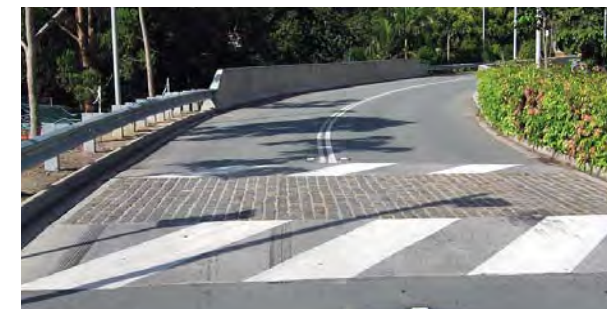
Raised pedestrian crossings that include textured pavers, colour and line marking are often used to highlight and mark the informal pedestrian crossing as separate from the road.
