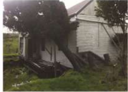
Damage to house due landslide
