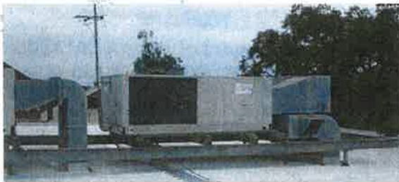
Main air conditioning units for new section (viewed from 1 st floor roof)
