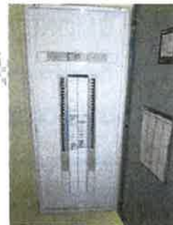
Photo: Carinó's Main Switchboard
