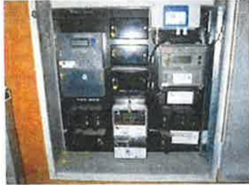
Photo: Main Switchboard with Metering
