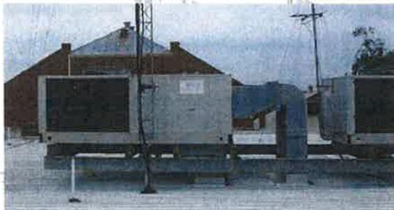
Main air conditioning units for extension section (viewed from 1 st floor roof)
