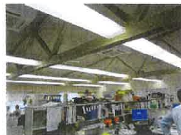
Photo: Office Lighting
