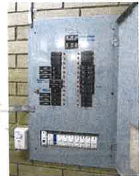
Photos: Curves Switchboard
