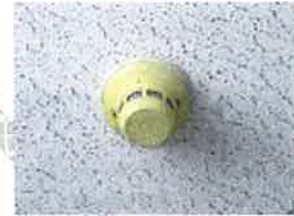
Photo: Smoke Detector (Unknown manufacture)
