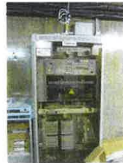
Photo: Telstra Optical Fibre
