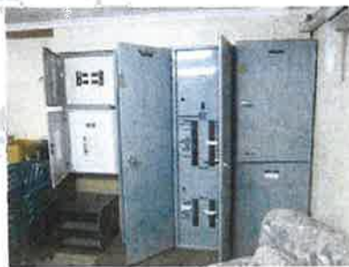
Photo: Main Switchboard
