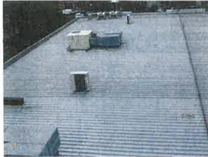
Main air conditioning units for original section (viewed from 1 st floor roof)
