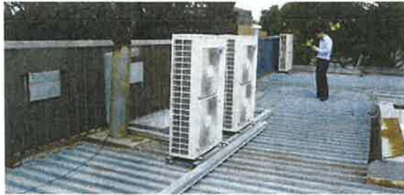
Carino's Building – Three air conditioning units for main office area (photo above) and two more air conditioning units for main office area (photo below) (all condensing units on roof) N.B. some capping on the top of the walls is quite rusted.
