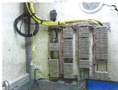
Photo: Main Distribution Frame
