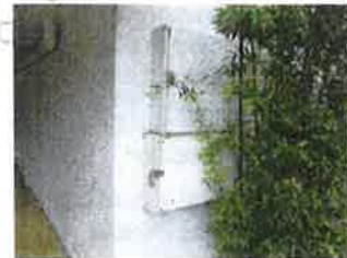
Photo: Outdoor Metering Enclosure
