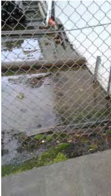
Poor stormwater management at 17 Ranceby Road causes rainwater to course across the surface of walkways and driving areas.
