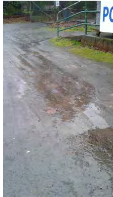
Spilling stormwater is clearly evident making its way across walkway and driveway sections.
