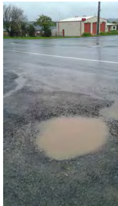
Potholes are everywhere!
