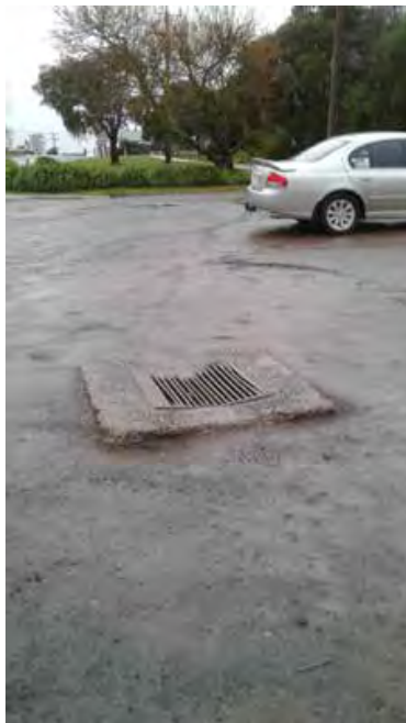
The potholes are matched only by the ugliness of the protruding stormwater pits which are treacherous for vehicles.
