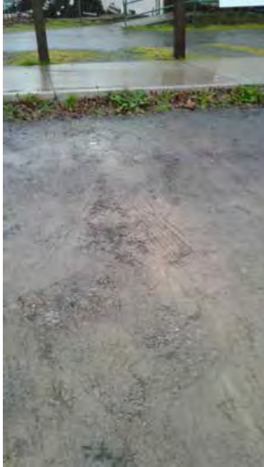
This pothole has been wearing for so long the clay has come to the surface of the stone.
