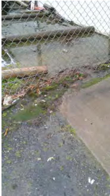
Walkway to the shops' entrances is particularly bad during wet weather. The first steps would be the lack of maintenance at 17 Ranceby Road which has caused many problems and safety hazards.
