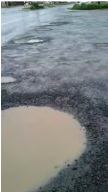
Cavernous potholes make access unsafe and unsightly.
