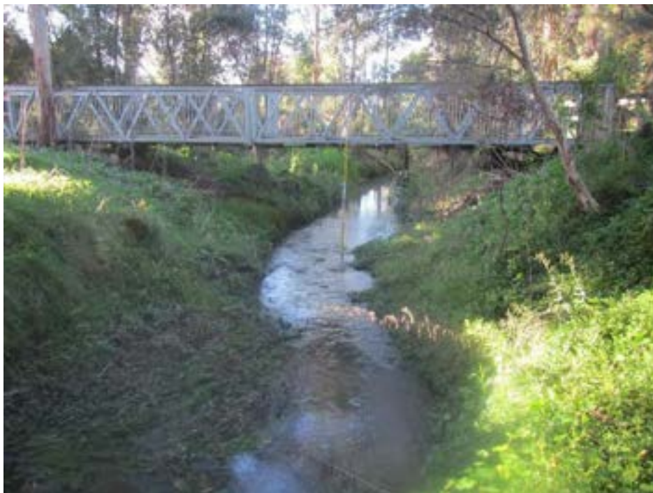
Appendix Figure A. 4 Pedestrian bridge adjacent to Foster Primary School – Stockyard Creek
