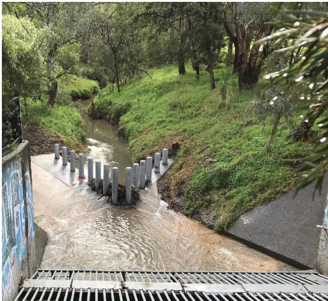
Figure 6.9 Steel bollards installed at Rosanna Parklands to prevent debris from entering drainage network
