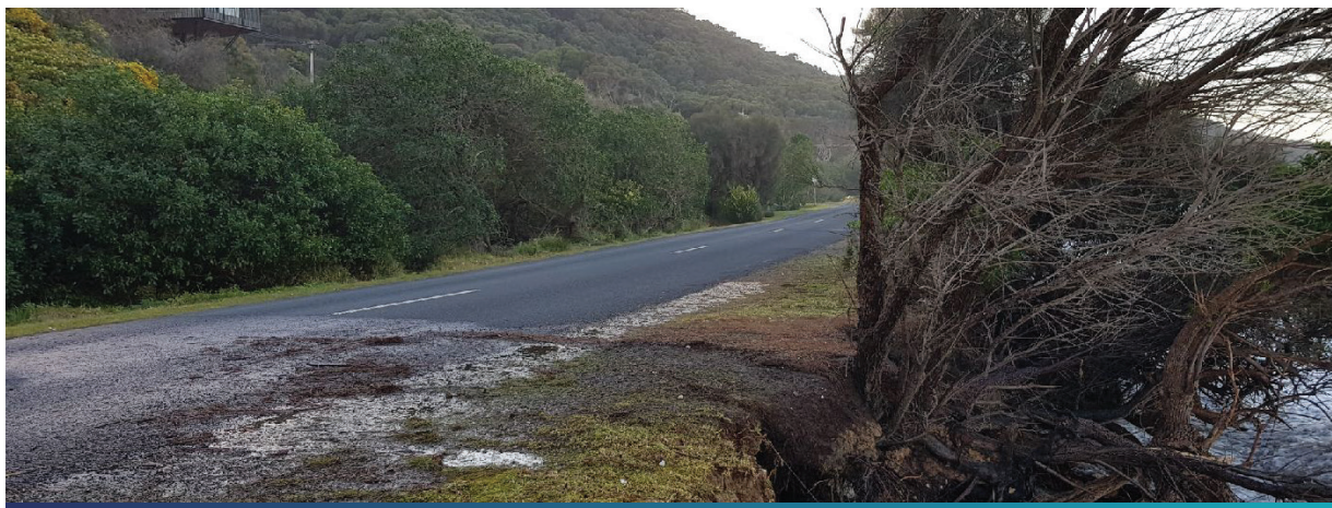
Wave erosion undermining road – Walkerville
