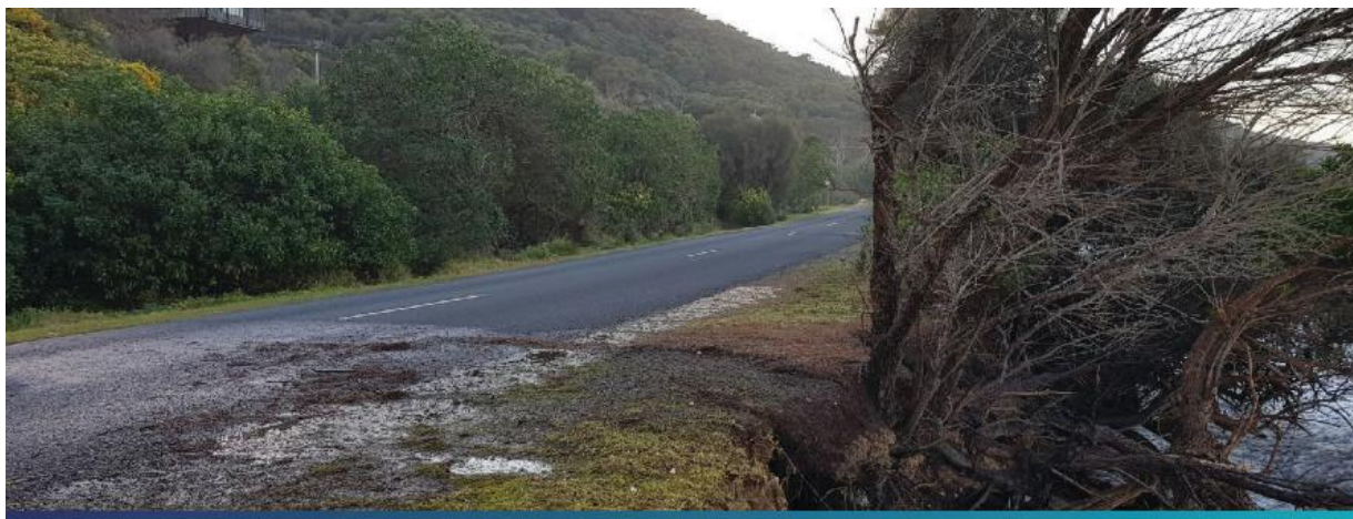
Wave erosion undermining road – Walkerville
