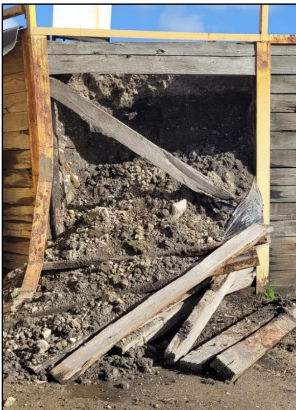
Figure 1 – Walkerville Transfer Station Failed Retaining Wall
