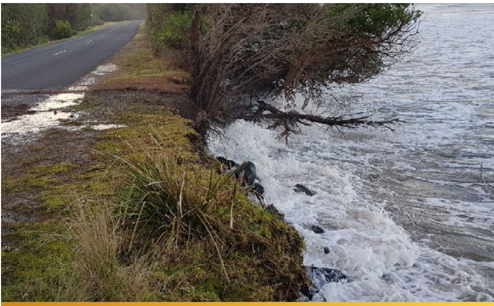
Large swells impacting roads at Walkerville – 2018
