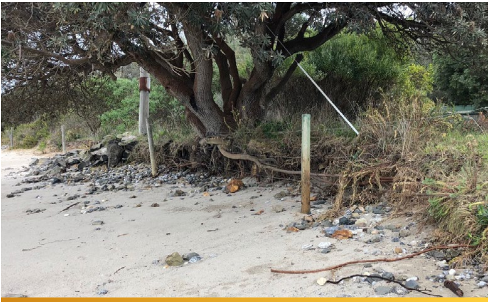
Erosion at Walkerville foreshore – after 2018 storms
