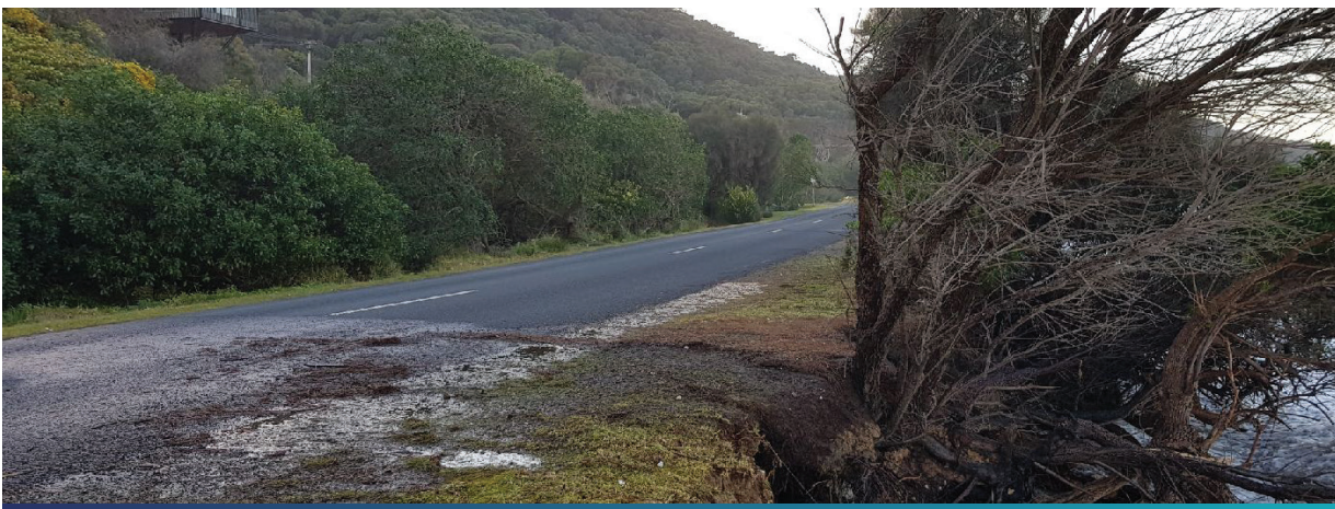
Wave erosion undermining road – Walkerville
