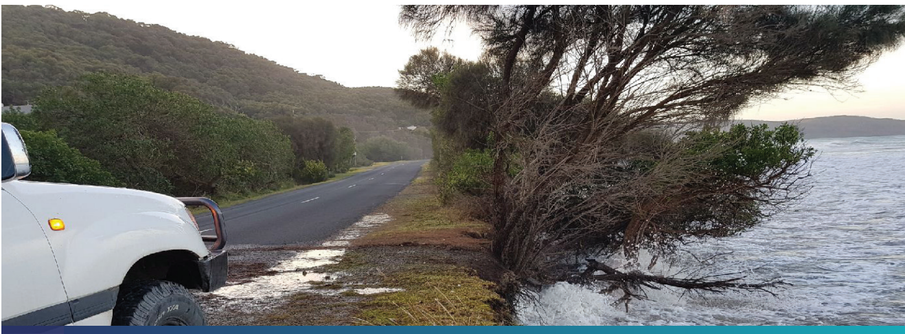
Wave erosion undermining road – Walkerville
