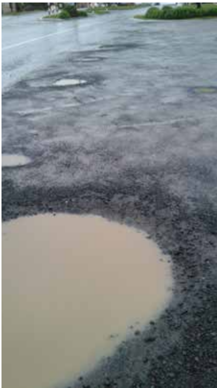
Cavernous potholes make access unsafe and unsightly.
