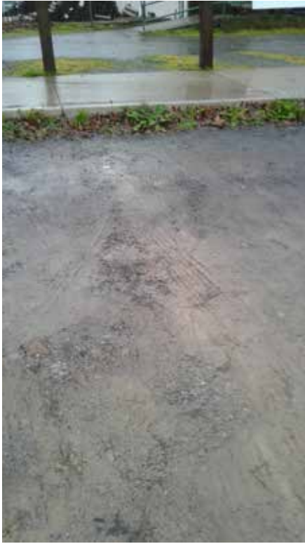
This pothole has been wearing for so long the clay has come to the surface of the stone.
