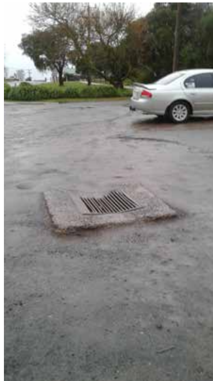
The potholes are matched only by the ugliness of the protruding stormwater pits which are treacherous for vehicles.
