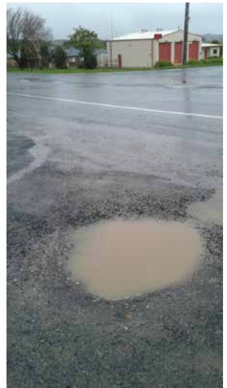
Potholes are everywhere!
