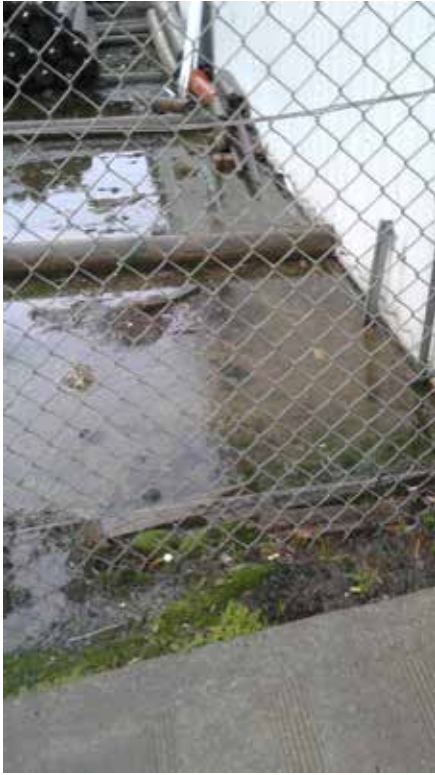
Poor stormwater management at 17 Ranceby Road causes rainwater to course across the surface of walkways and driving areas.
