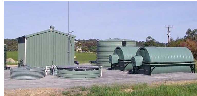
Figure 13. Typical arrangement of a RBC treatment plant - KBR, Fish Creek Sewer Study, 2014
