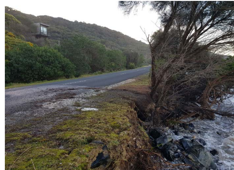
Erosion at Walkerville North
