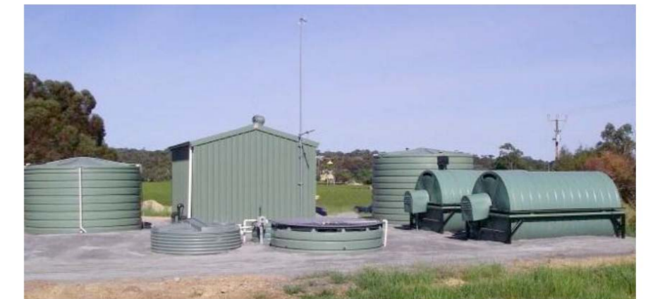
Typical arrangement of a RBC treatment plant - KBR, Fish Creek Sewer Study, 2014
