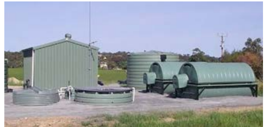
Figure 13. Typical arrangement of a RBC treatment plant - KBR, Fish Creek Sewer Study, 2014
